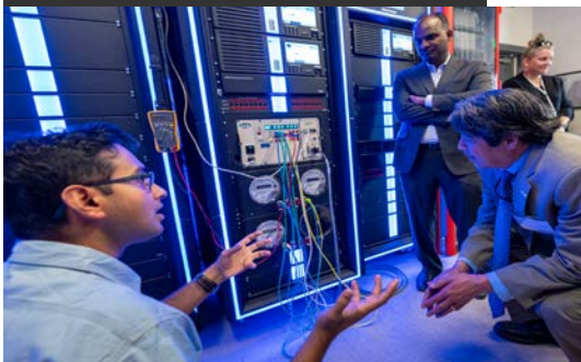
Photo by Werner Slocum NREL 78586
